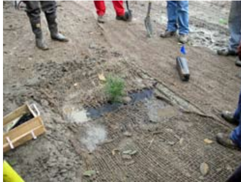
The thing that saved our bacon - some what was the thick fiber mat that had been laid down the day before by staff members of the Stream Restoration Alliance.
